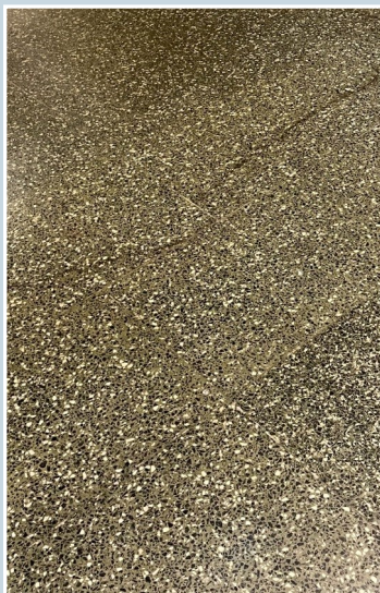
This is what the floors in our hallways looked like before scraping off the wax.
